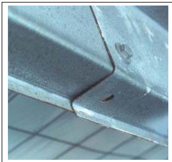
Figure 2. Early cut-edge corrosion on these continuously galvanized purlins – the thicker the section, the greater the risk of cut edge corrosion.
