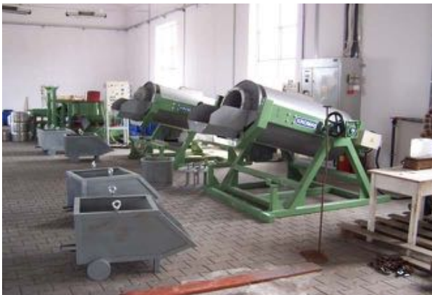
Small scale ArmorGalv® system – fits into a 100m 2 (1100ft 2 ) facility.
